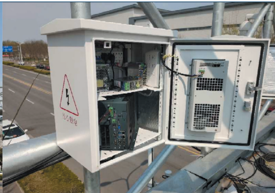
Figure 5. Deployment scenarios of Roadside MEC Equipment (in roadside cabinet).
