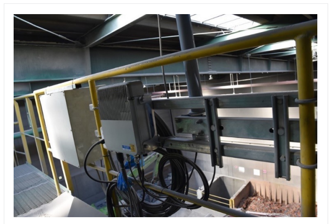
Figure 5. Location of local 5G equipment in the plant.
